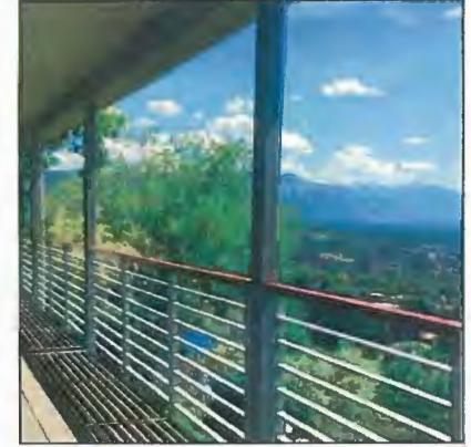
STEEL RAILING SYSTEM
